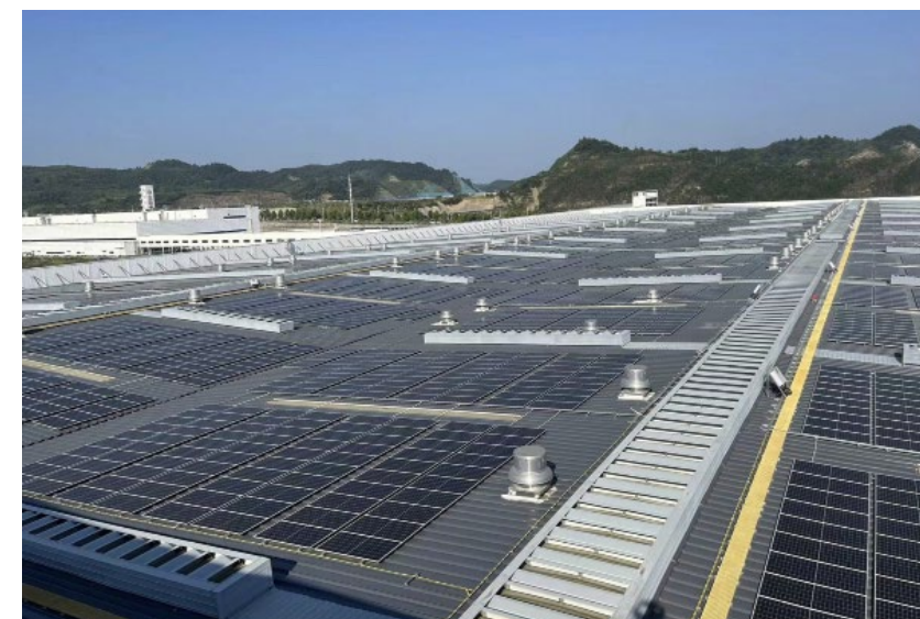
↳ Rooftop photovoltaic devices installed for warehouses
