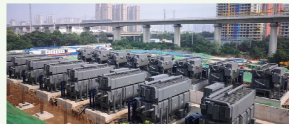
16 sets of 60MW lithium bromide heat exchange units
