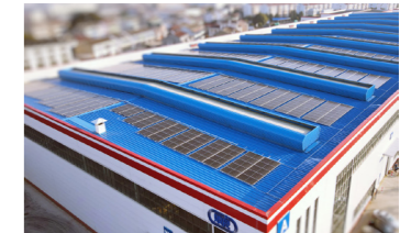
PV roof of the Company's factory
