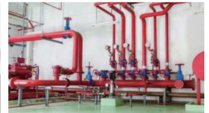
Fire Fighting Engineering
