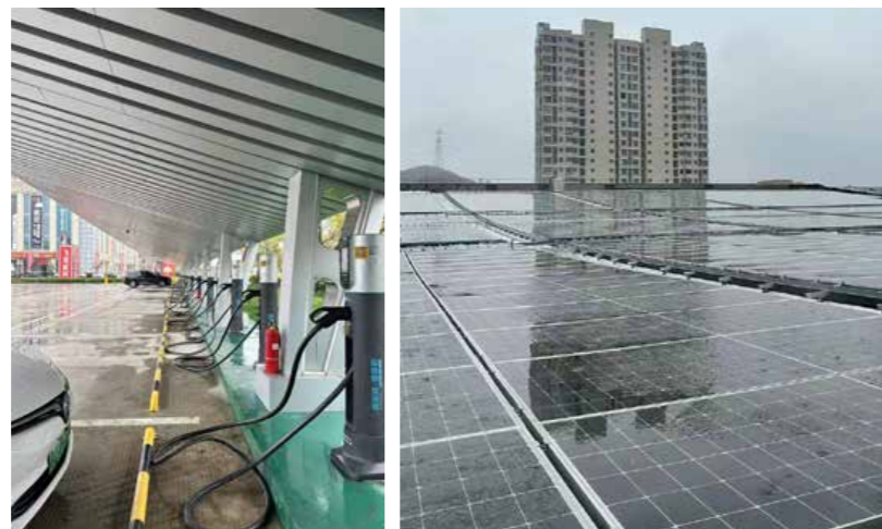
Assisting in demonstration project of the rooftop distributed photovoltaic and new energy vehicle photovoltaic storage and charging of Yuhuan Commercial Exhibition Center in Taizhou
