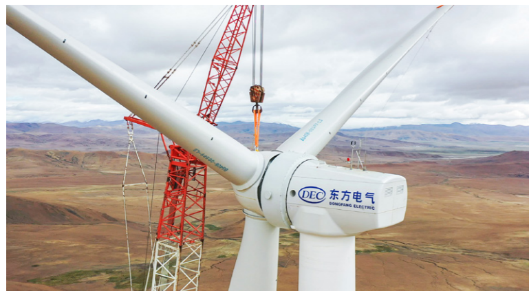
◀东方电气为世界最高海拔风电场——西藏措美县哲古分散式风电项目提供的 5 台 2.X-131 型永磁直驱超高海拔风电机组全容量并网发电 5 DEC 2.X-131 permanent magnetic direct drive wind turbines applicable to regions of ultra-high attitude were put into grid-connected power generation at full capacity in the world's highest-altitude wind power project—a distributed wind farm located at Zhegu, Cuomei County, Tibet
