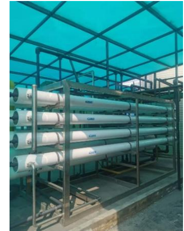
Washing water concentration treatment system
