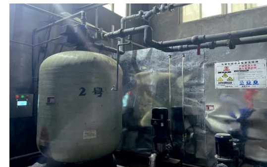
Waste heat water tank
