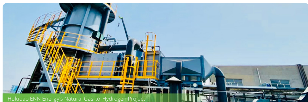
Huludao ENN Energy's Natural Gas-to-Hydrogen Project
