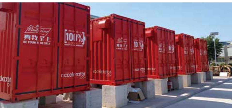
A container-based peak-shaving and valley-filling electrochemical energy storage power station project financed by the Bank
